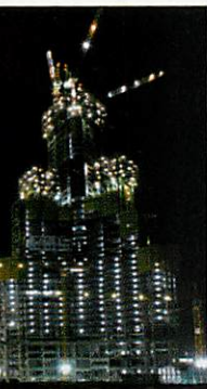
TALL WONDER: Construction of Burj Dubai at night. It will be the world's tallest building (2,650 feet) when complete.
